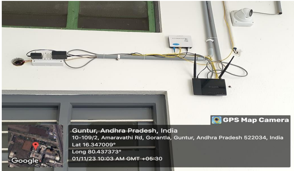
Wi-Fi router at Skill development Lab
