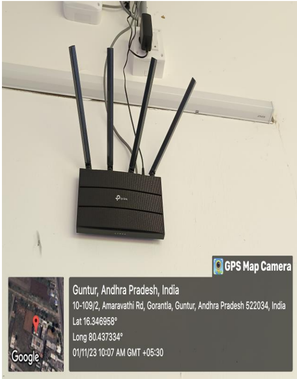
Wi-Fi router at Corridor
