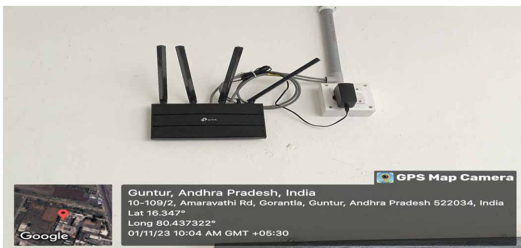
Wi-Fi router at Corridor
